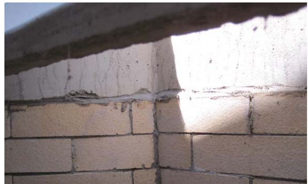
Figure 9. Back Walls of Throat Sitting Flush with Fire Brick
