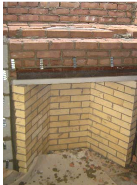
Figure 10. Building Up the Masonry to Create a Setting Surface for the Damper and Smoke Dome
